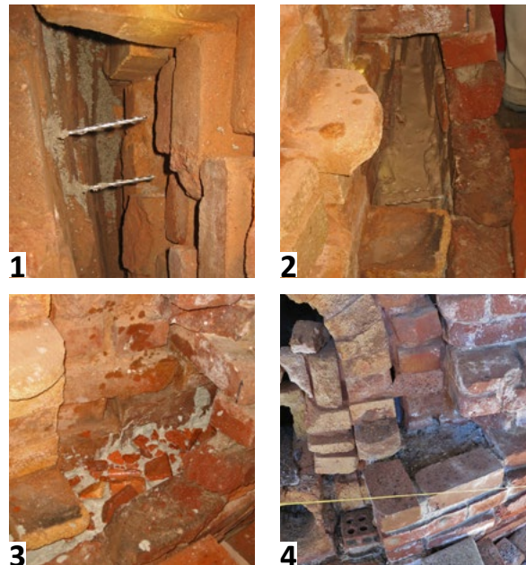
Matero leads the students (left) in a grouting demonstration seen step-by-step above. The void in the masonry is cleaned and prepared with stainless steel helical screws for added post-set strength (1). The grout is introduced—a composition of equal parts NHL 3.5 and sand mixed in a one-to-five part ratio (by volume) of SikaLatex acrylic fortifier and water (2). Brick fragments help fill the void (3), leaving a solid mass within a day's time (4).
