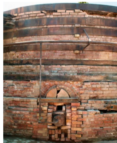
Summer Progress: Images of the northeastern portion of Kiln No. 7, before (above) and after (below) its initial stabilization in early July 2012.
