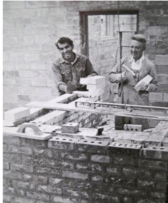
"Lots of Brick to Lay": Peter Voulkos (left) and Branson Stevenson at work with Western Clay brick and tile in 1951. The pottery's original downdraft kiln, which the two men are constructing above, was based on a design by Archie Bray himself. Source: Archie Bray Foundation Archives
