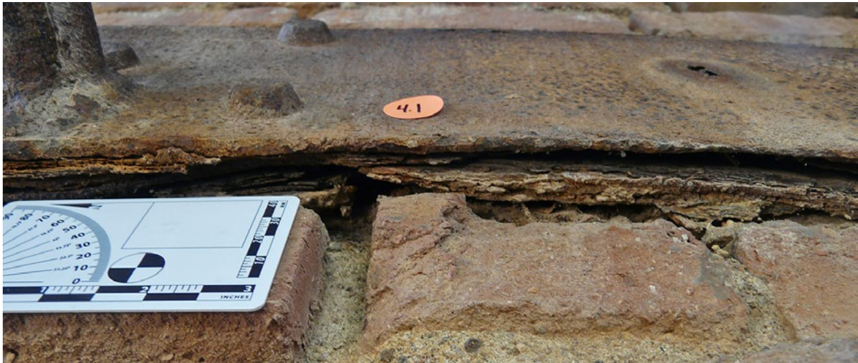
Heavy Metal: Layers of packing corrosion had built up between the kiln's steel bands and chloride-ridden brick walls, exerting a massive tensile force on whatever sound metal remained. Photo: K. Wohlgemuth
