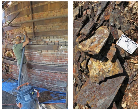
Paul Mardikian assisted with the arduous clean-up of corroded steel (bottom left and right). Chemello, meanwhile, prepared test treatments on bands retrieved from the other kilns (above).
