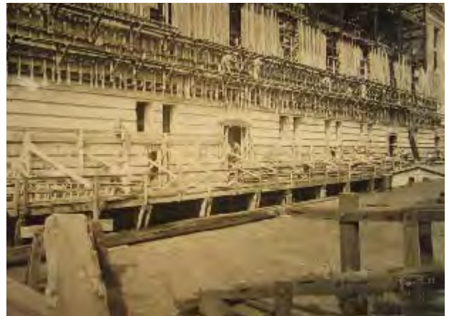
Figure 15: Construction of the Delaware Station, showing use of reinforced concrete, Photo c.1923. Source: PECO Archives.
