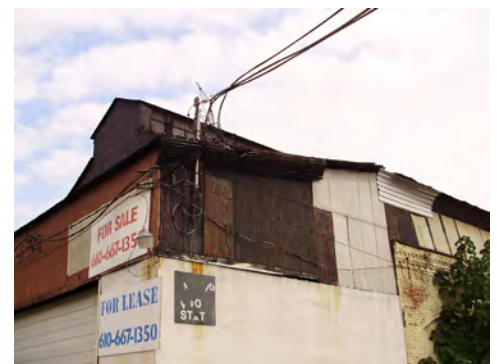
Fig. 5.2.19: Typical ferrous staining on Building 2.
