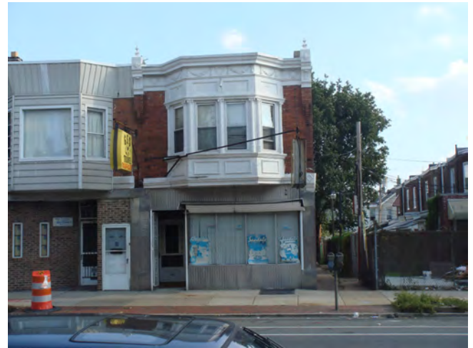
Fig. 5.3.13: This image, of 6807 Torresdale Avenue, exhibits many of the issues observed in the commercial area. To the left, a major first floor façade renovation closes the exterior to the street while the vinyl siding above covers architectural details at the cornice line. To the right, historic details are maintained at the second story, but the first floor window projects an unwelcoming façade with the addition of a roll-down window protection.
