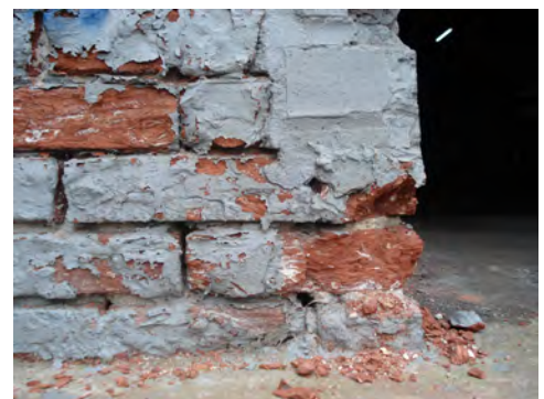
Fig. 5.2.17: Typical friable brick and mortar loss found along base of industrial buildings.
