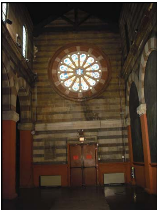
Figure 6.6.1. Soiling on south elevation of Sanctuary, 2009. Credit: by the authors
