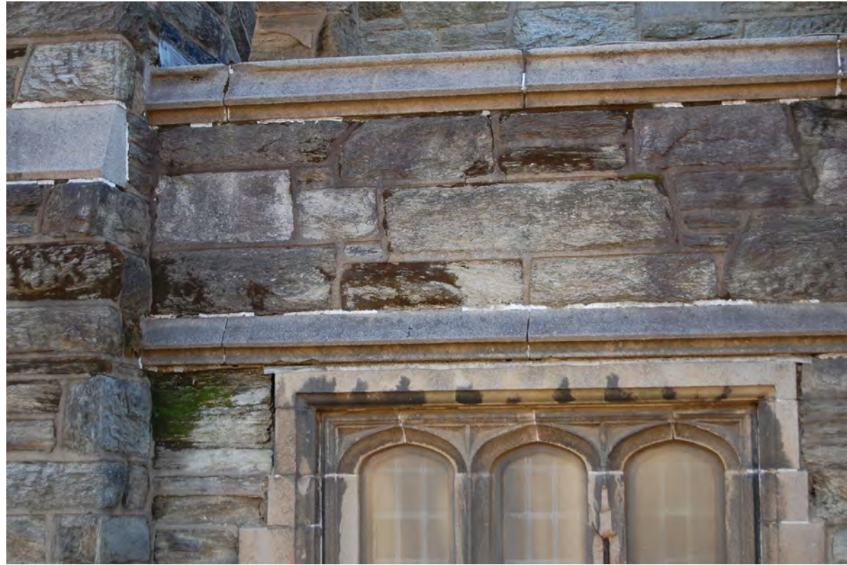
Figure 3 Biological growth, moisture staining, and inappropriate repointing on north elevation
