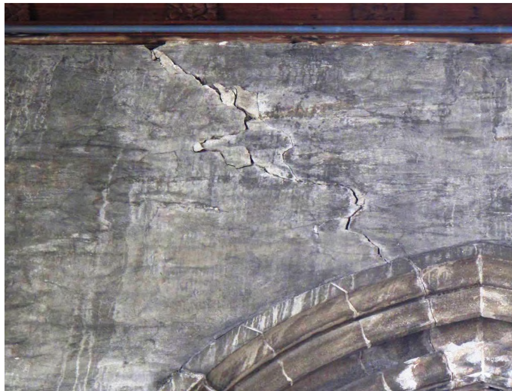
Figure 9 Crack on top of wall
