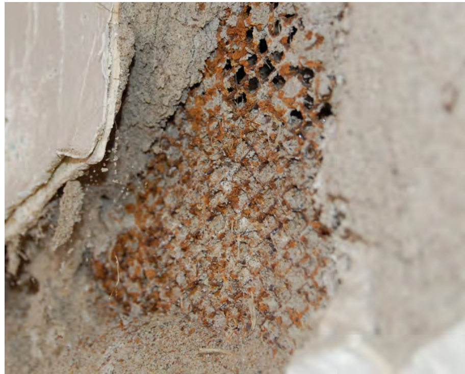
Figure 8 Failing metal lath and plaster system
