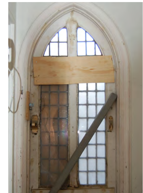
Figure 2 Door in very poor condition on the Deanery leading to courtyard
