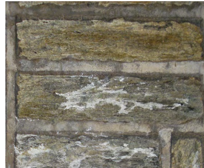
Figure 6 Severely deteriorated schist in the interior of the Chapel
