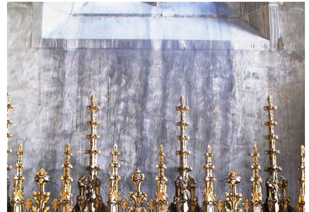
Figure 8 Water staining on cement stucco wall.
