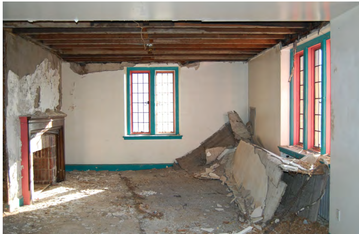
Figure 13 Collapsed plaster ceiling in southwest room, second floor
