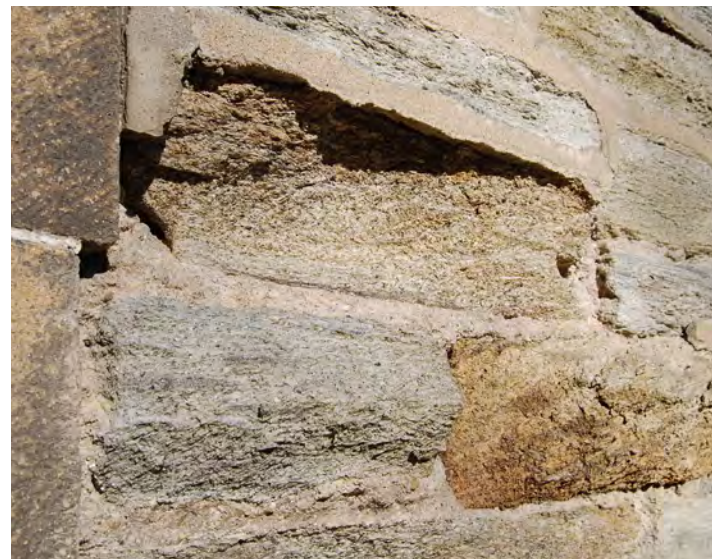
Figure 4 Severely deteriorated schist on the exterior
