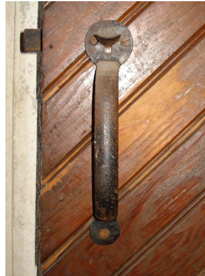
Figure 10 Interior door showing rusted hardware and loss of wood finish
