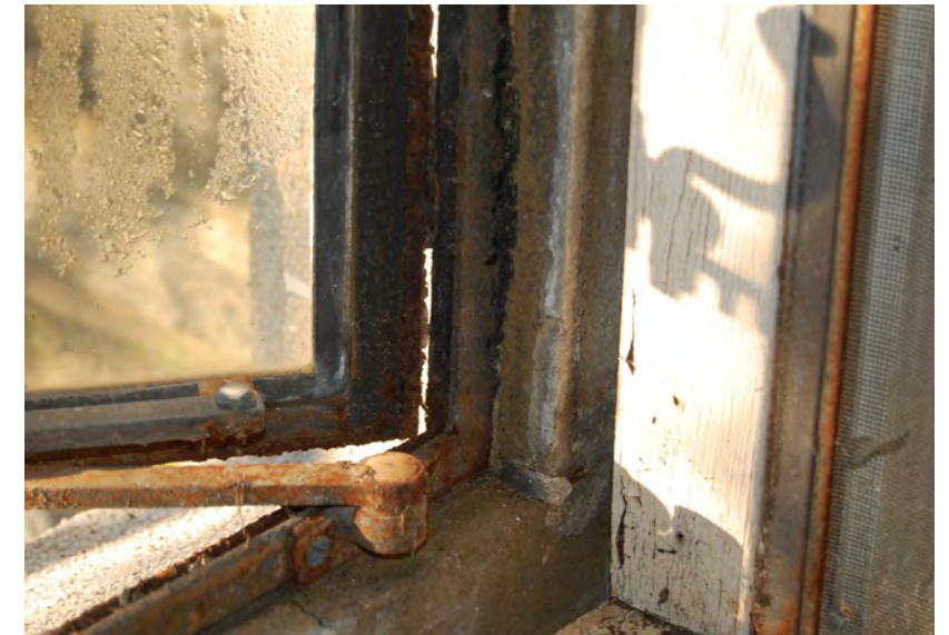
Figure 4 Rusting of frame and subframe
