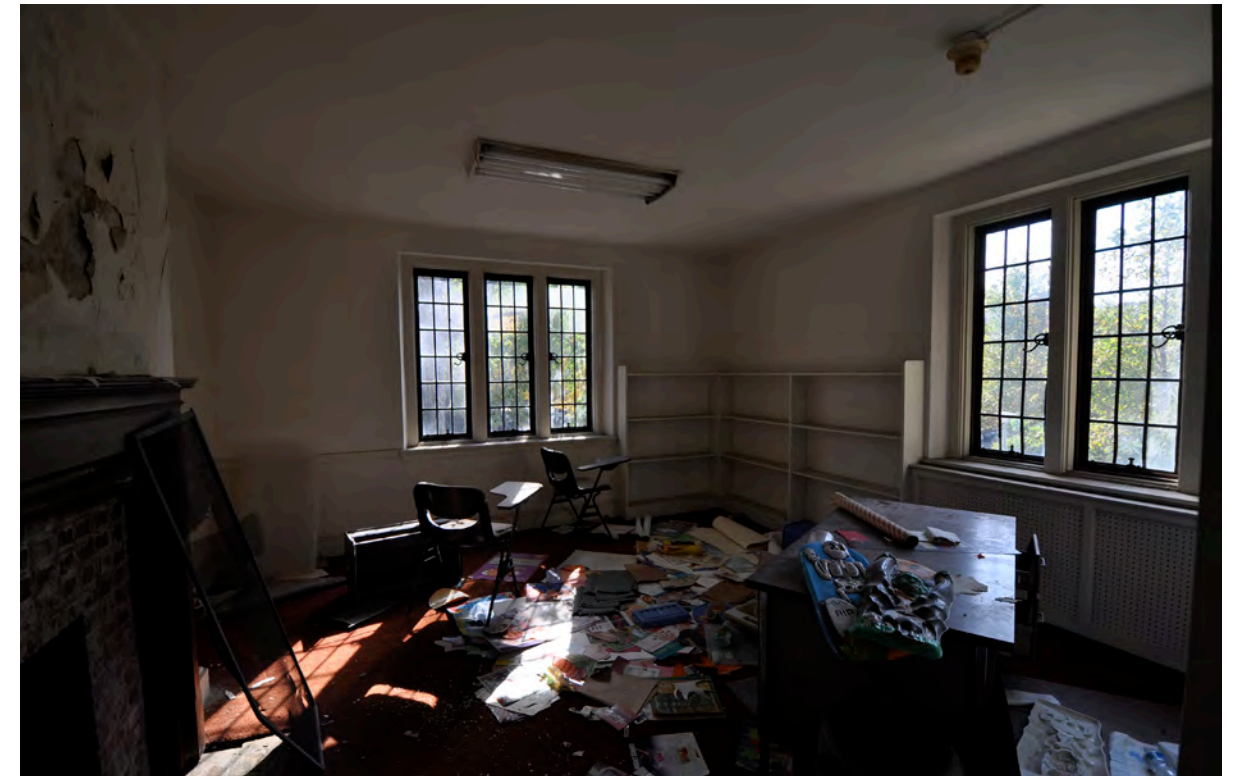
Figure 3 View of the condition of one of the rooms on the second floor of the Deanery
