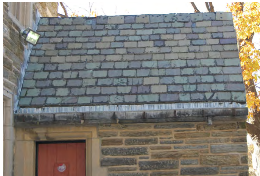
Figure 1 Section of St. Andrew's roof showing, chipped, cracked, broken, and delaminating slates.
