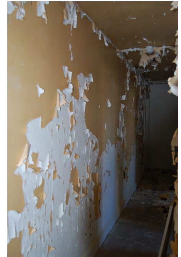
Figure 14 Peeling paint in third floor hall of deanery
