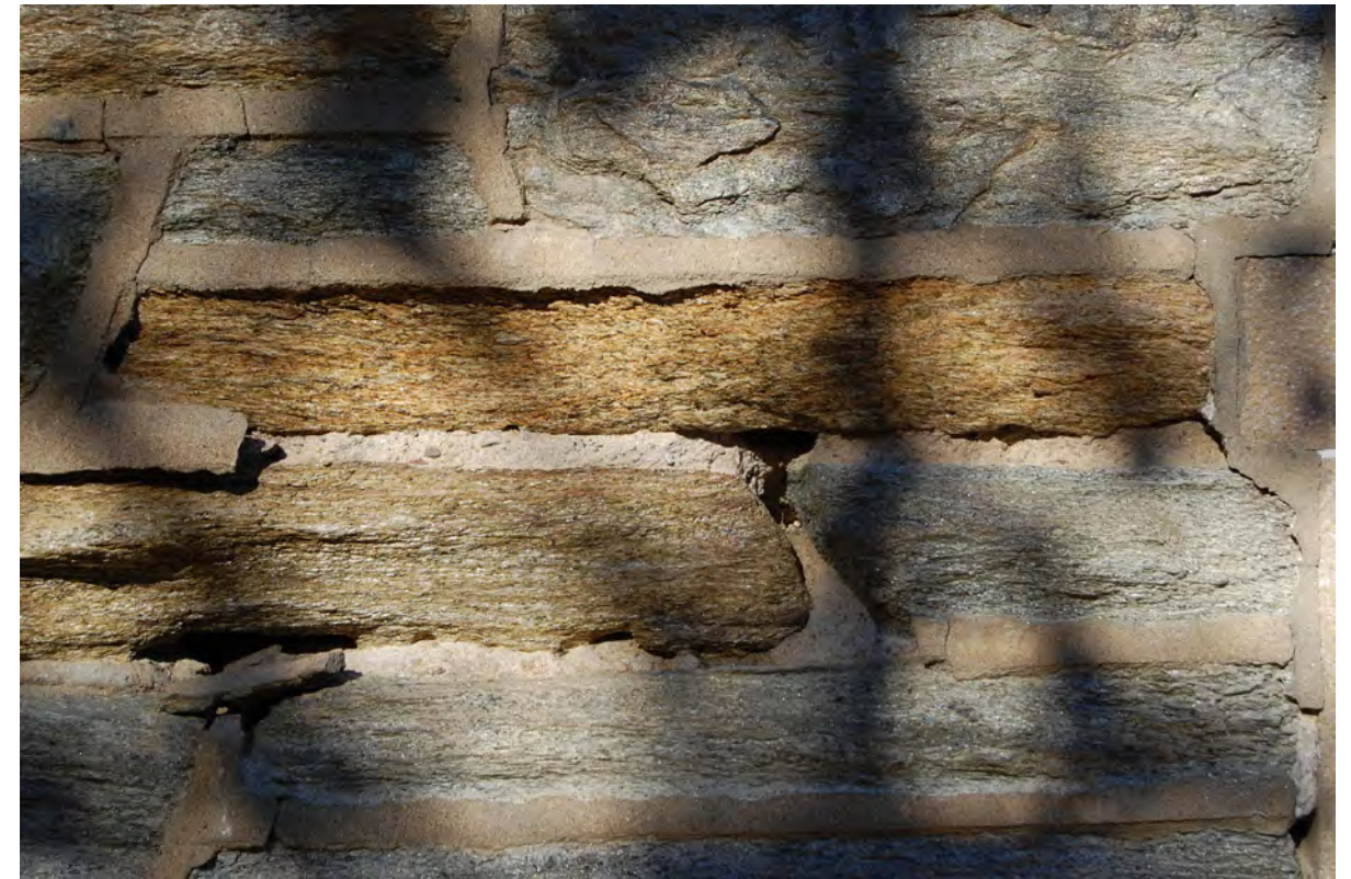
Figure 2 Deteriorated mortar and inappropriate repointing with hard Portland cement mortar
