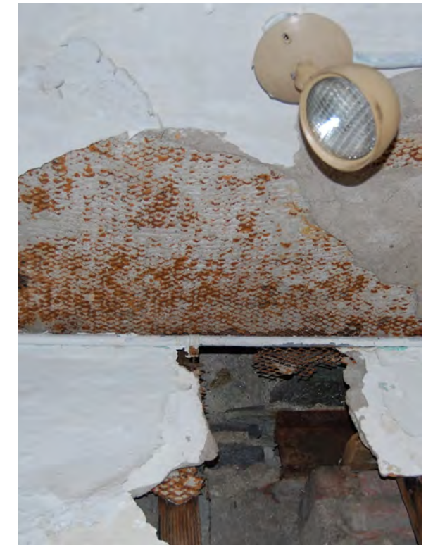
Figure 2 Deterioration surrounding plaster and metal lath in the deanery
