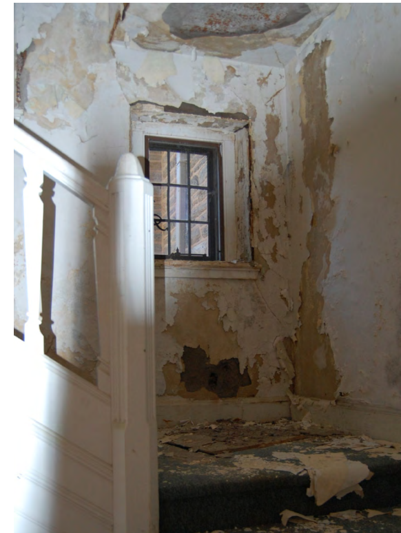
Figure 1 General deterioration surrounding a window in the Deanery
