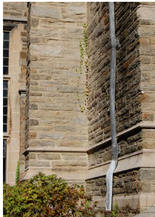
Figure 7 Failing downspout, southwest corner of chapel
