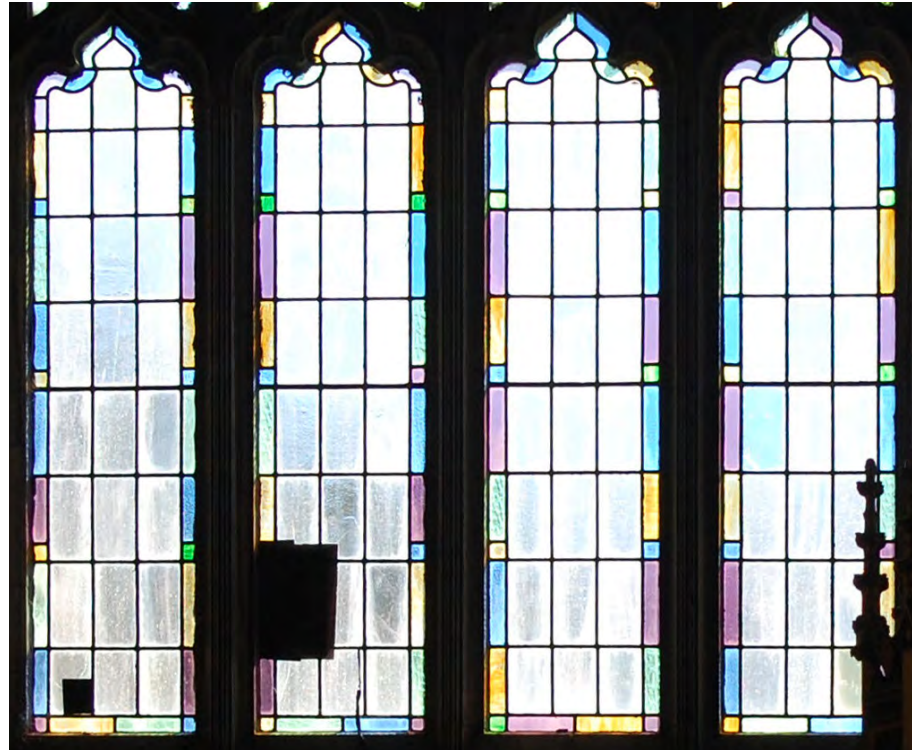
Figure 7 Missing glazing on south end of the Chapel
