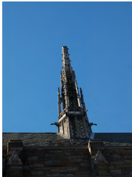
Figure 6 Flèche, top third removed due to structural problems
