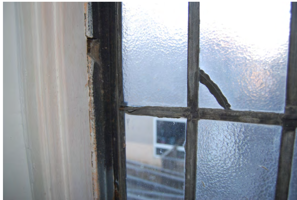
Figure 3 Deterioration of lead comes
