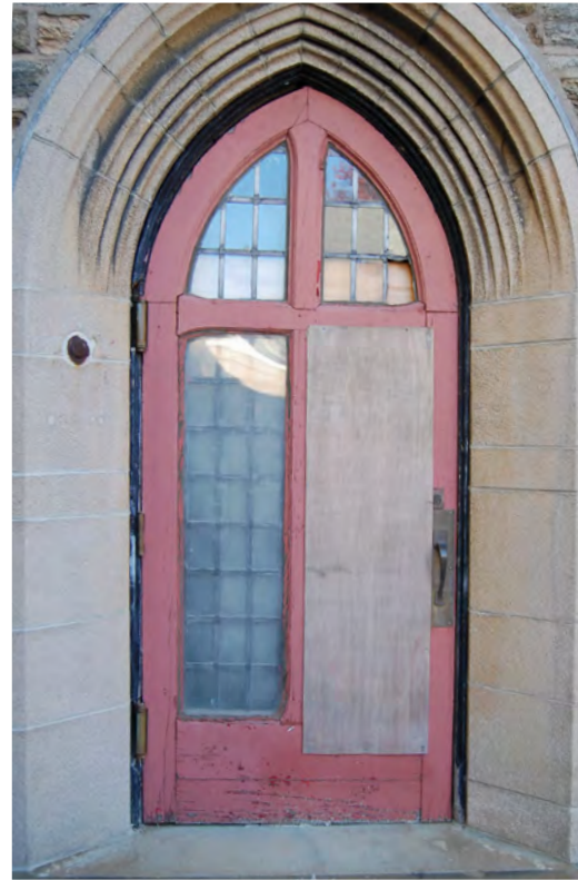
Figure 5 Vandalized deanery door
