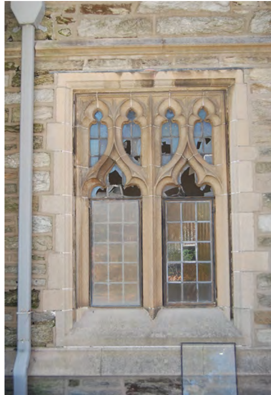
Figure 4 Broken glass, east ambulatory window
