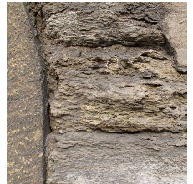
Figure 3 Salt deposits, likely gypsum, have formed a crust over stones on the southern elevation.
