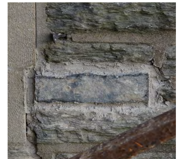
Figure 6 A second inappropriate replacement on the western elevation of the Deanery.
