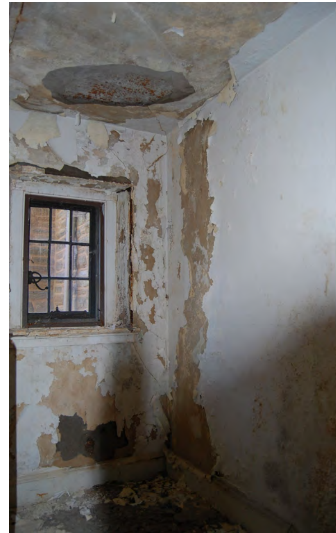
Figure 12 Plaster and finish deterioration due to water damage
