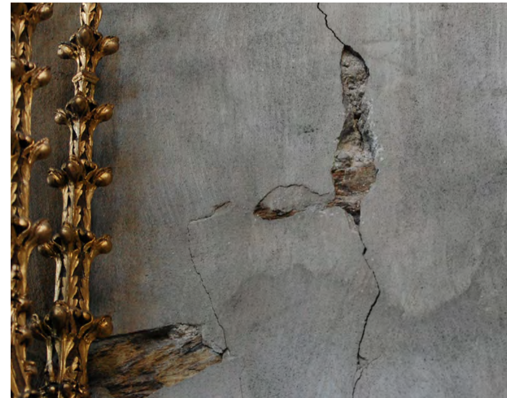
Figure 9 Cracks and cement detachment on walls
