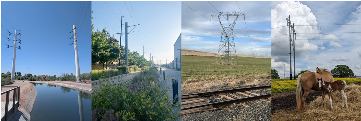
Figure 1. Examples of transmission ROW colocation 1 examples. From left to right: canal-site multi-use path (SPR PERA facility, AZ, credit Rebecca O’Neil); urban greenway within a city power corridor (Salt Lake City, UT, credit Emma Hibbard); transmission line parallel to the Hartline-Coulee City rail line (WA, credit Irena Netik); and horses grazing under a transmission line (Campbellsville, KY, credit Rebecca O’Neil)
