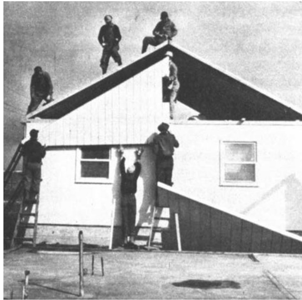
Figure 1. A building crew constructs a panelized National Homes house. (Source: "F.O.B.: Fifty Houses a Day." Fortune, April 1950, 94.)
