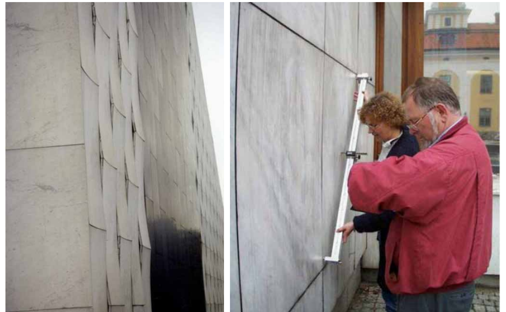
Figure 2(left). Part of the old marble facade at Finlandia Hall in 1999. (Source: Symposium on Dimension Stone Use in Building Construction Tampa, Fla). Figure 3(right). Measurements of bowing amplitudes with the use of a Bow meter. (Source: Symposium on Dimension Stone Use in Building Construction Tampa, Fla)
