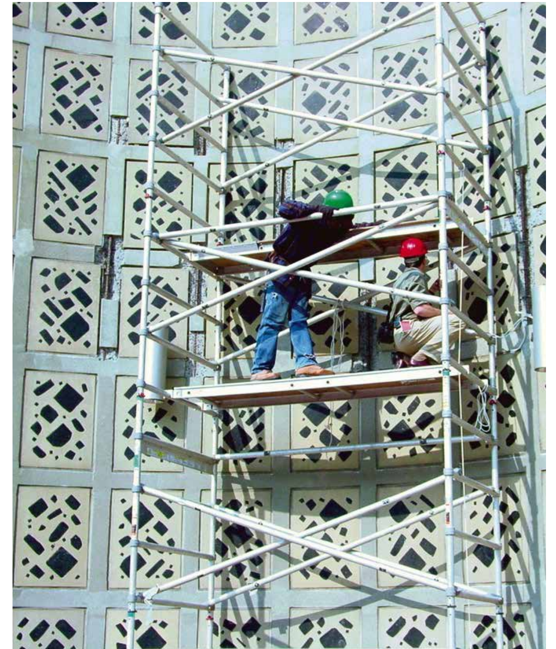
Figure 2. Conservation of dale-de-verre at the New York Hall of Science. (Source: Ennead Architects).
