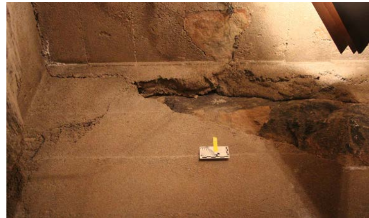
Figure 4.7 Cracks found across the desert masonry walls Image Credit: Authors, March 2023
