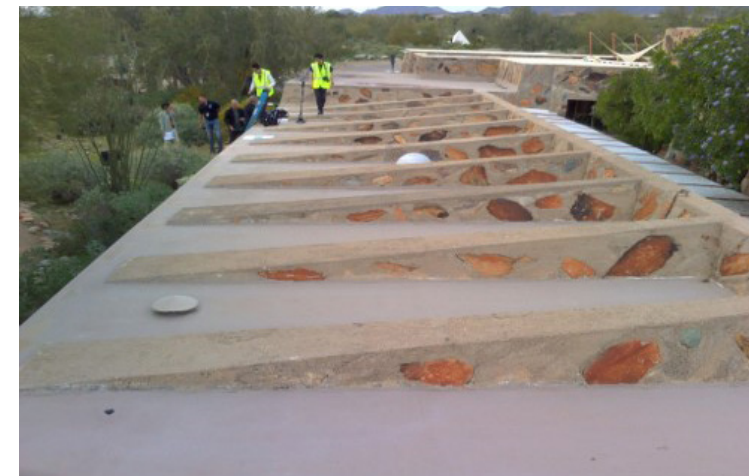
Figure 3.7 Image of the roof looking north showing the upturned beams. Image Credit: Author, March 2023
