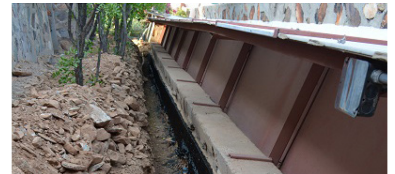
Figure 2.24 2014 waterproofing along the East wall Source: Frank Lloyd Wright Foundation Preservation Records
