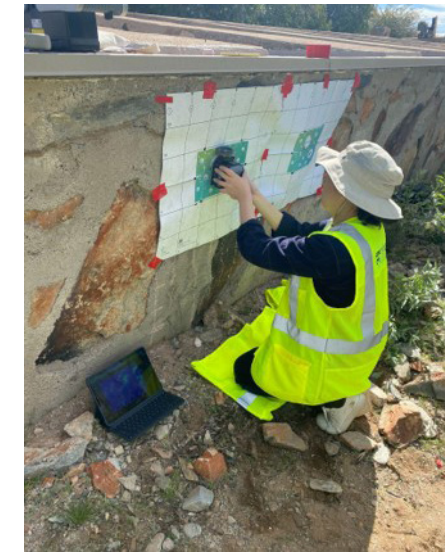
Figure 4.24 Student taking the GPR scan along the West wall Image Credit: Author, March 2023
