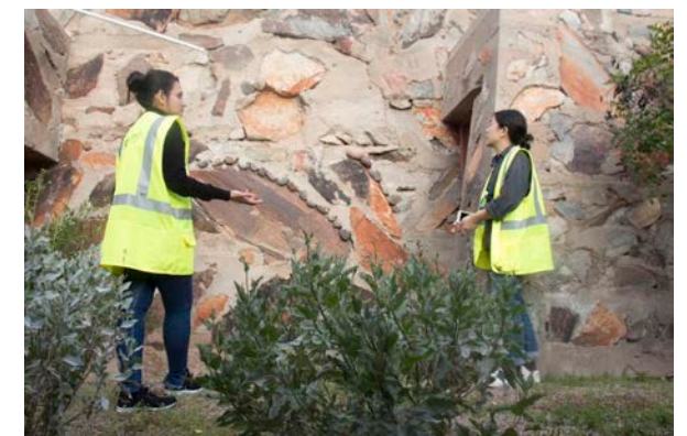
Figure 4.2 On-site documentation undertaken by students during their study trip Image Credit: Authors, March 2023
