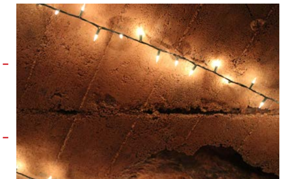
Figure 4.16 Photo taken from underside of the roof slab showing the exposed rebars Image credit: Author, March 2023
