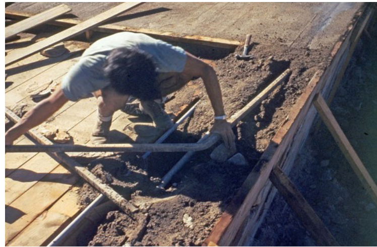
Figure 4.21 1948 construction photo of the roof showing the X-pattern rebar anchoring into the end slabs along the West end. Source: Frank Lloyd Wright Foundation Archives
