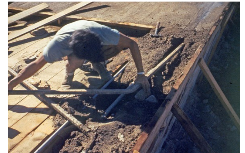
Figure 3.8 1948 construction photo of the roof showing the X-pattern rebar anchoring into the end slabs along the west end Source: Frank Lloyd Wright Foundation Archives
