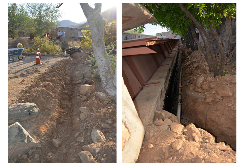
Figure 4.5 Waterproofing campaign undertaken by the Frank Lloyd Foundation in 2014 Image Credit: Frank Lloyd Wright Foundation
