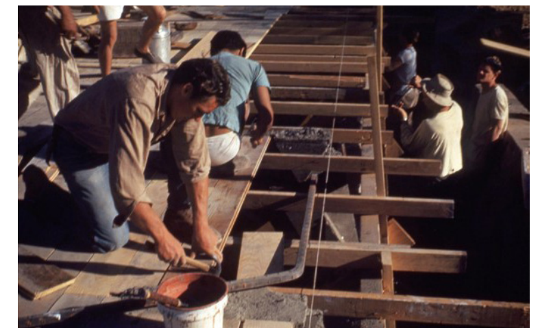
Figure 3.9 1948 construction photo of the roof showing the X-pattern rebar anchoring into the end slabs along the east end. Source: Frank Lloyd Wright Foundation Archives
