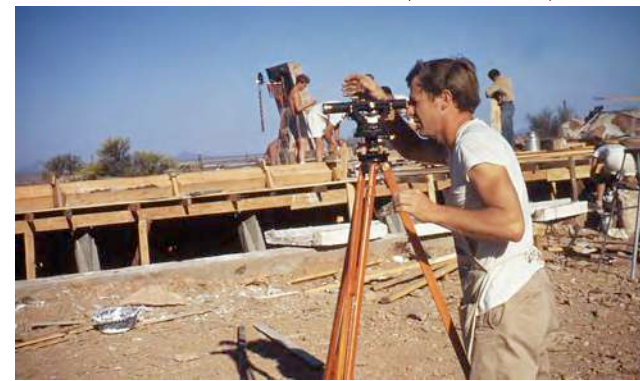
1948-1949 Construction of Cabaret. (Source: Taliesin West Archive, "Construction Taliesin West" historic photo collection.)
