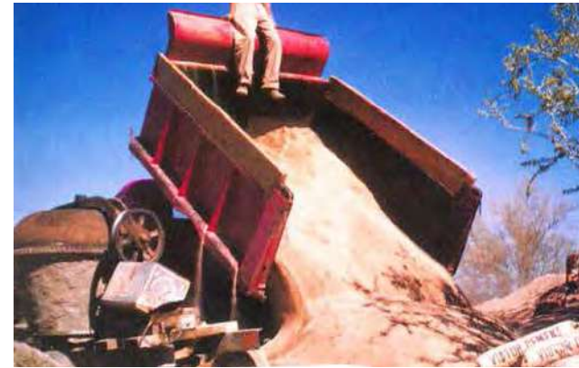
1948-1949 Unloading the sand at the cement-mixer. (Source: Gottlieb, Lois Davidson. A Way of Life: An Apprenticeship with Frank Lloyd Wright. I. publ, Images Publ, 2001.)
