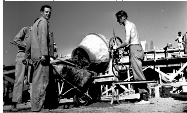
1947 Wes Peter (left) Construction at Taliesin West. (Source: Taliesin Fellowship – Pedro E. Guerrero. https://guerreroportfolio.com/portfolio/taliesin-fellowship/ .)
