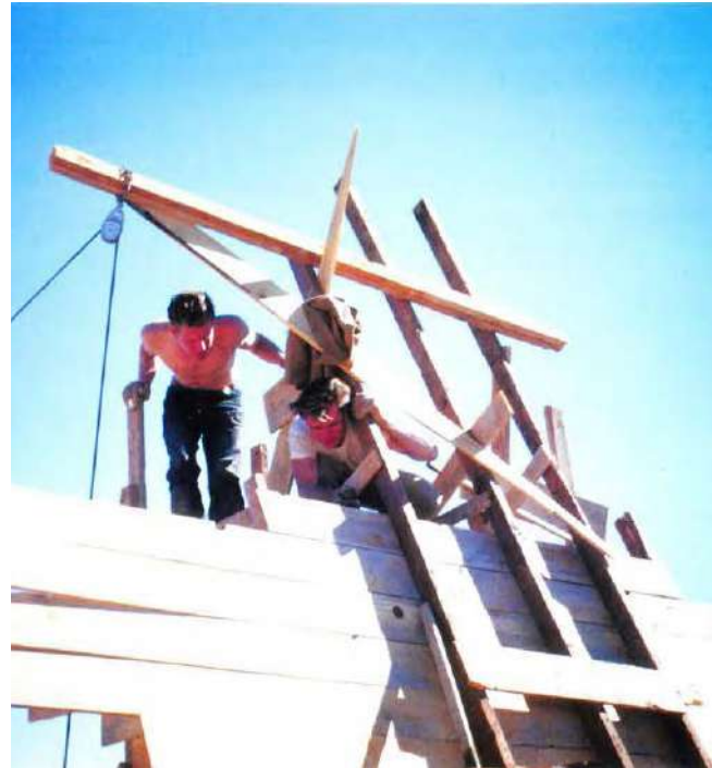
1948-1949 A close-up of the chimney construction. (Source: Gottlieb, Lois Davidson. A Way of Life: An Apprenticeship with Frank Lloyd Wright . I. publ, Images Publ, 2001.)
