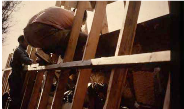
Typical wall construction (Source: Taliesin West Archive, "Construction Taliesin West" historic photo collection.)
