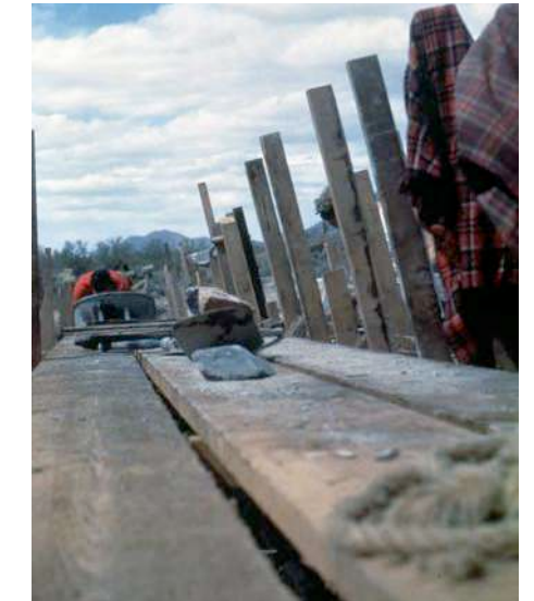
Wall construction (Source: Taliesin West Archive, "Construction Taliesin West" historic photo collection.)
