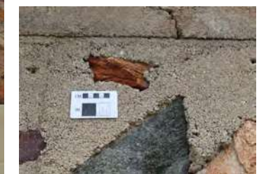
cold joint concrete texture
