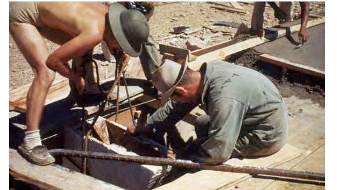
1948-1949 Wes Peter and Joe Fabris lowering the forms into place. (Source: Taliesin Fellowship – Pedro E.Guerrero. https://guerrerophoto.com/portfolio/taliesin-fellowship/ .)
