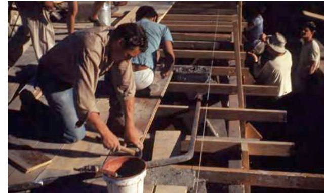
1948-1949 Construction of Cabaret concrete roof. (Source: Taliesin West Archive, "Construction Taliesin West" historic photo collection.)
