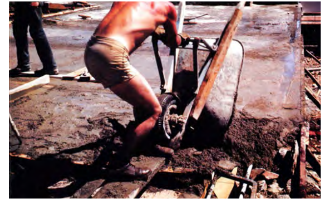
1948-1949 Tony Capucelli delivering the concrete. (Source: Taliesin Fellowship – Pedro E. Guerrero. https://guerreroportfolio.com/portfolio/taliesin-fellowship/ .)
