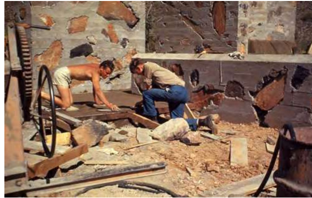
1949 Smoothing out and leveling the concrete floor at Taliesin West. (Source: Taliesin Fellowship – Pedro E. Guerrero. https://guerreroportfolio.com/portfolio/taliesin-fellowship/ .)
