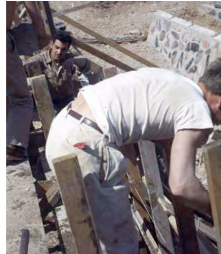
1963 Pavilion construction (Source: Taliesin West Archive, "Construction Taliesin West" historic photo collection.)
