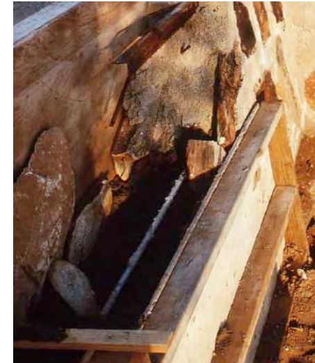
Wall construction (Source: Taliesin West Archive, "Construction Taliesin West" historic photo collection.)
