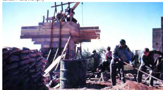
1948-1949 Building the chimney. (Source: Gottlieb, Lois Davidson. A Way of Life: An Apprenticeship with Frank Lloyd Wright. I. publ, Images Publ, 2001.)
