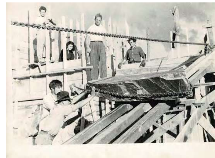
1944-1945 Taliesin construction (Source: Taliesin West Archive, "Construction Taliesin West" historic photo collection.)
