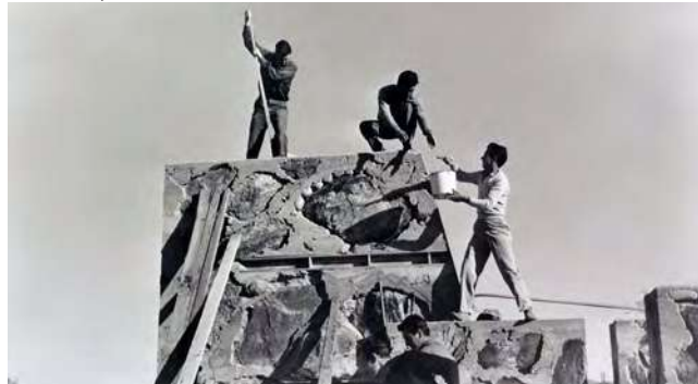
1956 Construction at Taliesin West, with apprentice Arnold Roy on right. (Source: Taliesin Fellowship – Pedro E. Guerrero. https://guerreroportfolio.com/portfolio/taliesin-fellowship/ .)
