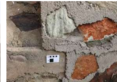
concrete color cold joint
