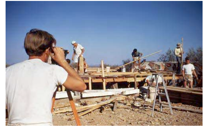
1949 Curtis Besinger surveying the roof for cabaret (Source: Taliesin West Archive, "Construction Taliesin West" historic photo collection.)
