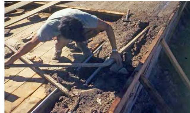
1948-1949 Construction of Cabaret concrete roof. (Source: Taliesin West Archive, "Construction Taliesin West" historic photo collection.)
