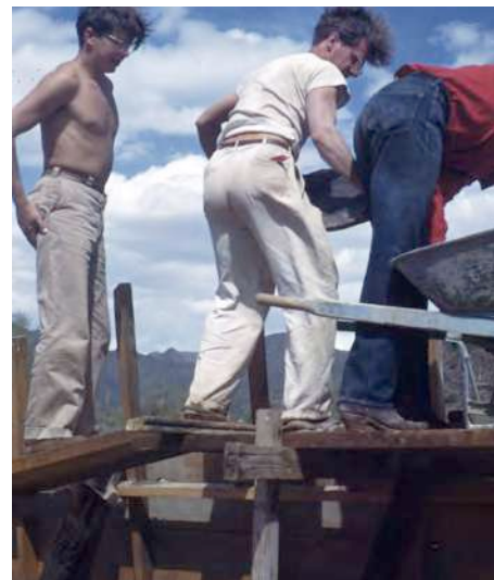
1963 Pavilion construction (Source: Taliesin West Archive, "Construction Taliesin West" historic photo collection.)
