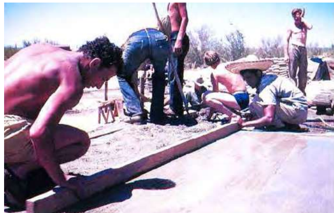
1948-1949 Fende Askill, from Turkey, screeding the concrete. (Source: Gottlieb, Lois Davidson. A Way of Life: An Apprenticeship with Frank Lloyd Wright . I. publ, Images Publ, 2001.)
