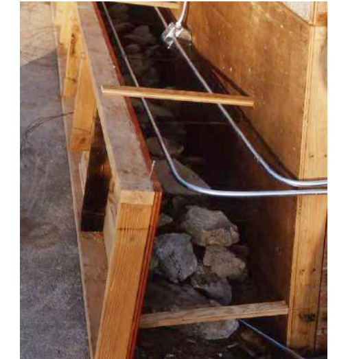
Wall construction (Source: Taliesin West Archive, "Construction Taliesin West" historic photo collection.)
