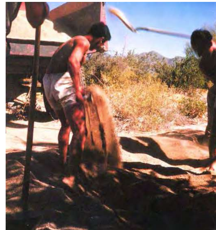
1948-1949 Sand was collected at a wash (a dry riverbed) in the desert, and used to make concrete. (Source: Gottlieb, Lois Davidson. A Way of Life: An Apprenticeship with Frank Lloyd Wright . I. publ, Images Publ, 2001.)
