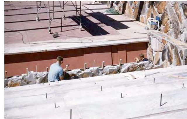
1963 Construction of Music pavilion stage (Source: Taliesin West Archive, "Construction Taliesin West" historic photo collection.)
