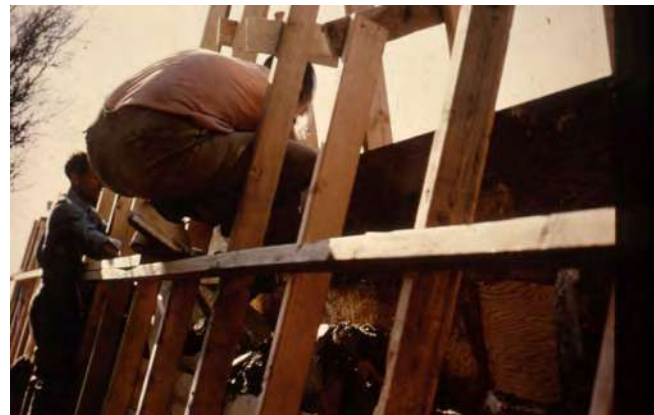
Figure 2.6. Placing stone into forms. (Source: Taliesin West Archive, "Construction Taliesin West" historic photo collection.)
