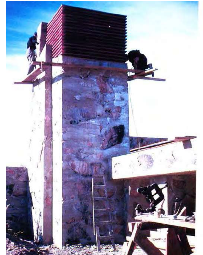
1948-1949 Apprentices putting the final touches on the water tower. (Source: Gottlieb, Lois Davidson. A Way of Life: An Apprenticeship with Frank Lloyd Wright . I. publ, Images Publ, 2001.)
