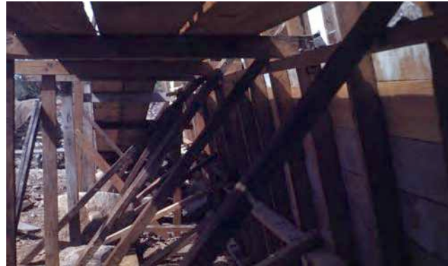
Wall construction (Source: Taliesin West Archive, "Construction Taliesin West" historic photo collection.)
