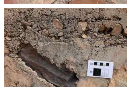
lifts, cold joint, honeycombing
